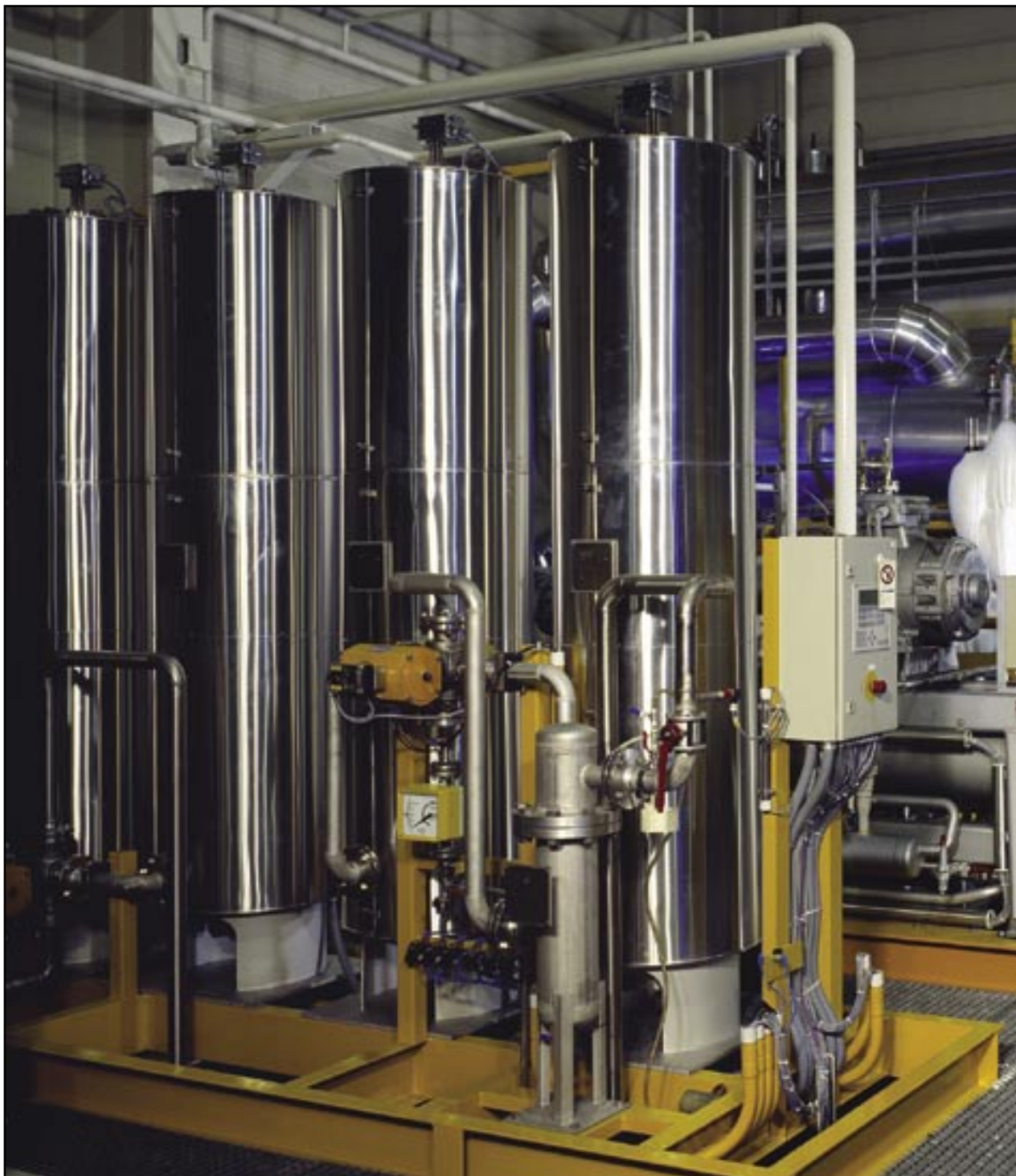
Activated Carbon Filter and Drying System.
